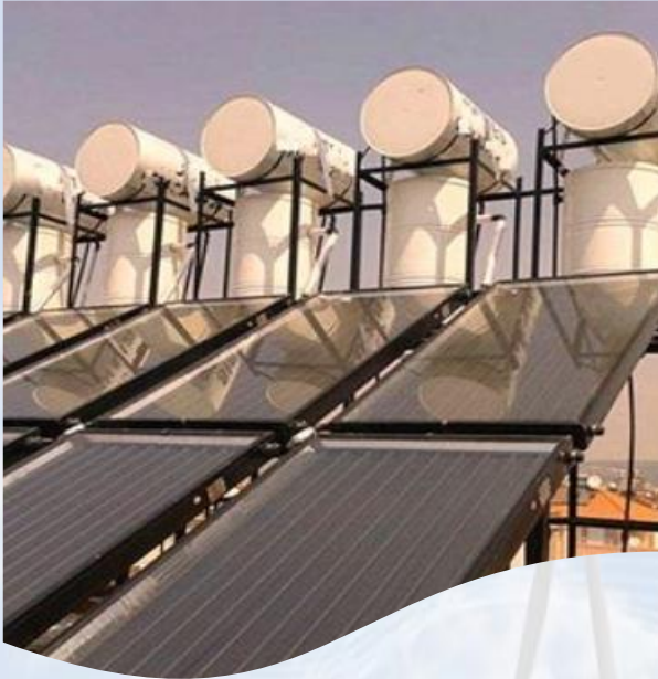
Roof Solar Heating Systems
