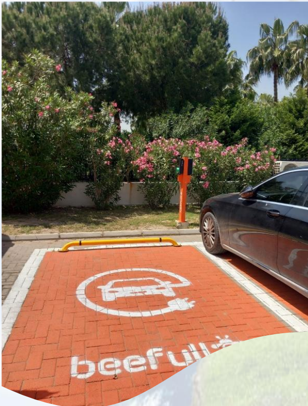
Electric Vehicle Charging Stations
